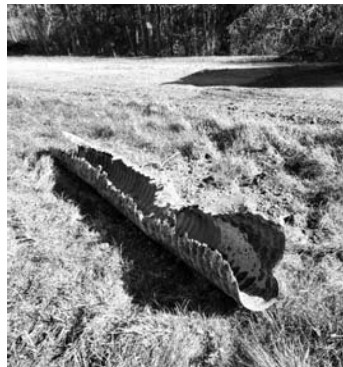
Cross pipe on Station Rd. Father time has had its way with this piece of pipe and the entire bottom has rotten away. A new HDPE pipe was installed in its place.
