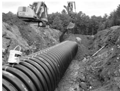
Crews working on West Old County Rd. installing a new 36 inch culvert to eliminate a trouble area that has caused road damage due to flooding and eliminated safety issues due to lack of access in the past.
