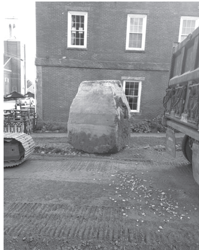
Figure 1A large concrete structure that was found in the roadway of Academy Hill. Items such as this were discovered up and down the roadway. Each one was addressed and corrected.
