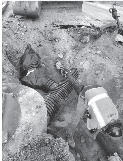
Figure 3 Crews working at the intersection of Academy Hill and Main St. Coordination with GSB Water Dist and MDOT was paramount on this project This picture shows new drainage being installed and new water line over the top of the drainage line.
