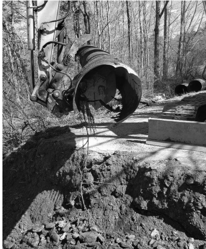
Failed culvert caused the road to give way on Kavanaugh Rd. Heavy rains washed a section of the road away prompting an emergency replacement. Note: bottom of the pipe had deteriorated to the point it no longer was present.
