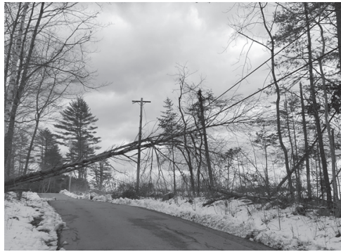
Storm damage on West Old County Road, one of numerous storms to have in impact this past year. Currently all debris has been removed and large tree stumps are scheduled to be picked up in the coming weeks.
