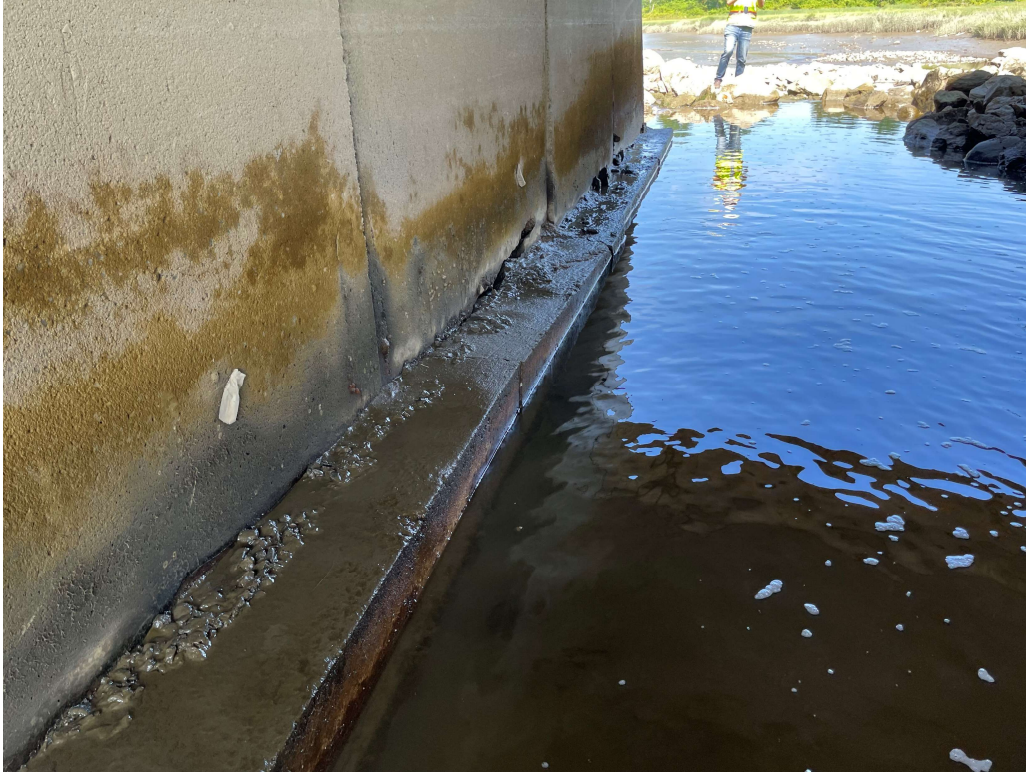
Southern damaged footing
