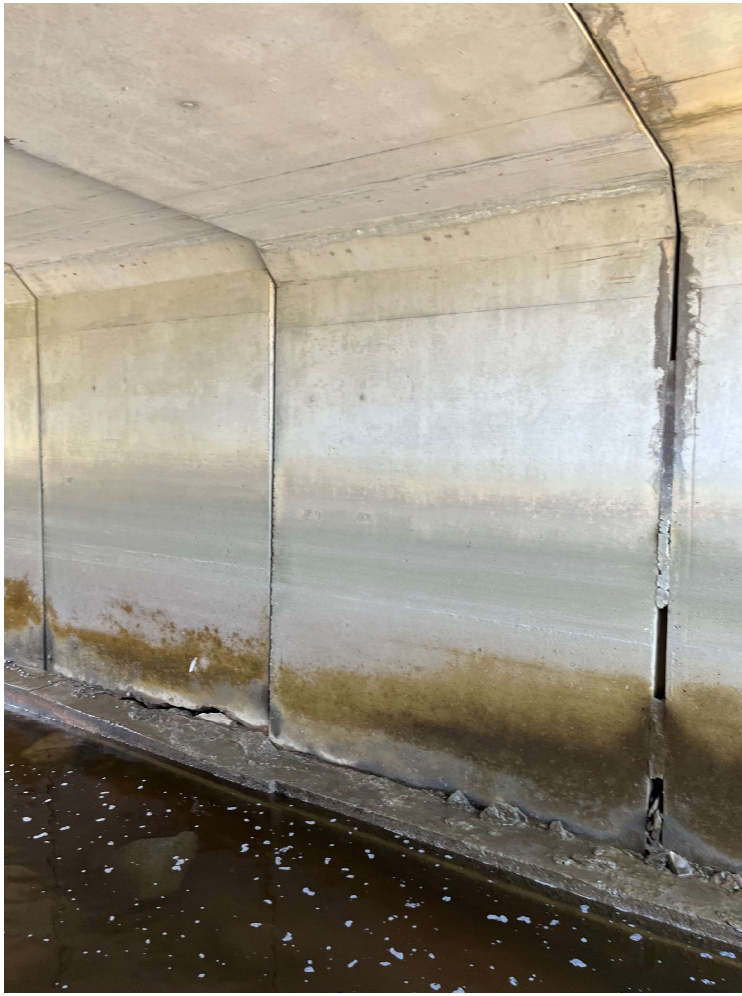
Separation of frame sections and footing damage
