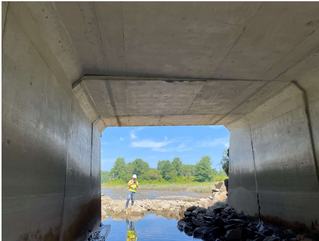
Distortion/Settlement of frame sections
