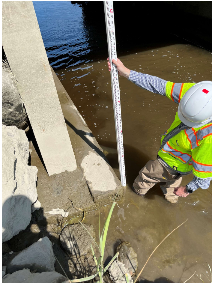
Exposed footing and undermining
