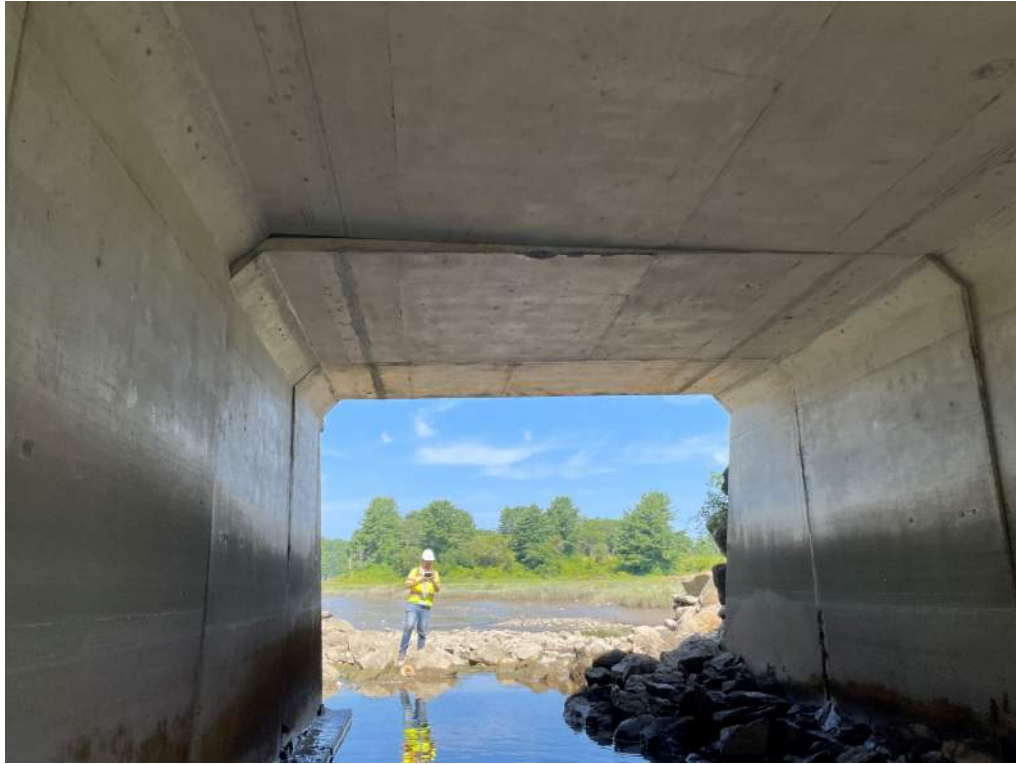
Photo 11: Key Feature: misaligned culvert section due to undermined footing
