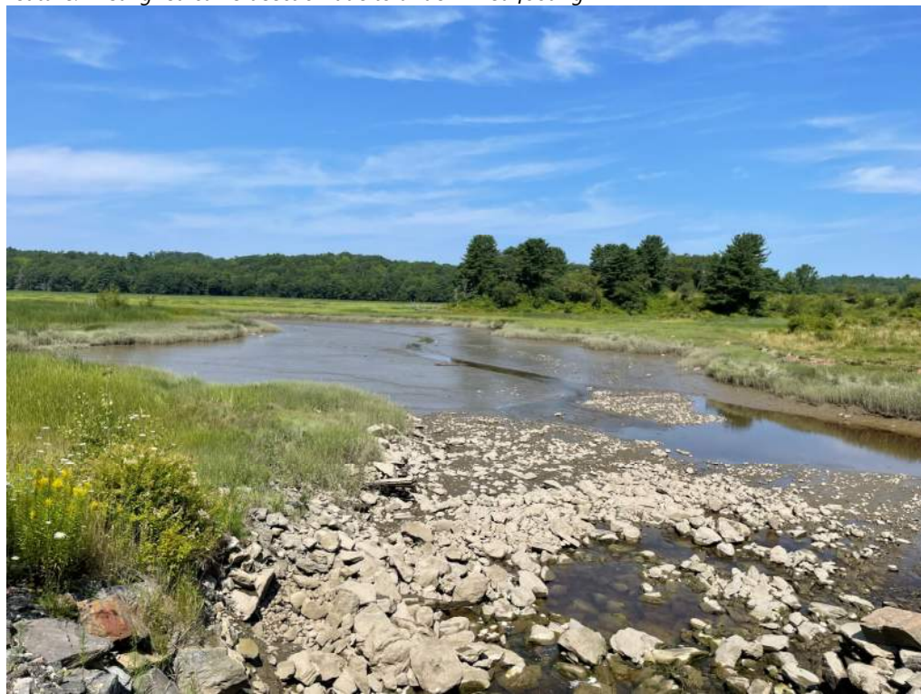
Photo 12: Key Feature: scattered deposits of riprap scoured from channel through culvert.
